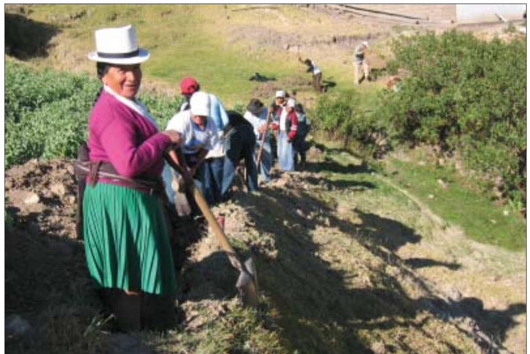
In Patadel, Ecuador, a volunteer crew of 130 men, women, and children dug a 650-m-pipeline trench, scheduled to take an entire week, in three hours, as part of a EWB project to improve the village water supply system. The community assisted EWB with spring source location, capture construction, water tank excavation, and water tank assembly. Photo by EWB-UMCP
