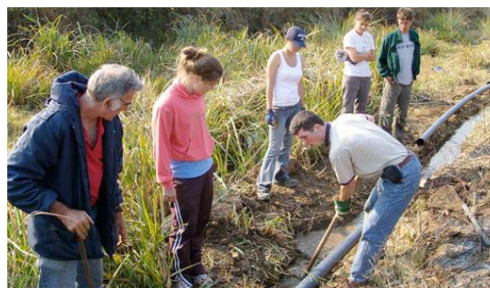
Dave Alcock supervises the team members as they prepare for the installation of the new ram pump system.
